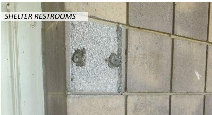
17 There is some damage, moisture infiltration and efflorescence to the exterior masonry
