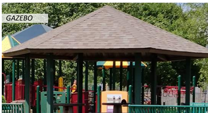
23 The shingle roof is in good condition, while the drip edge is fair
