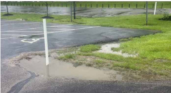
15 Parking experiences ponding and some drainage issues after heavy rains
