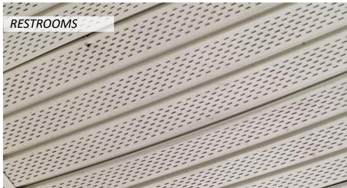
19 The soffit panels are sagging and there is evidence of moisture at base of masonry walls
