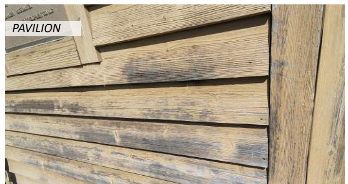
24 The wood finish is weathering and peeling, with columns beginning to delaminate
