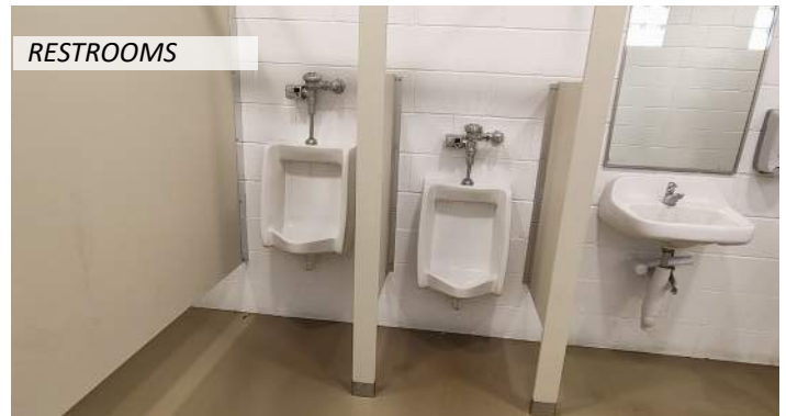
20 The restrooms lack proper accessible signage, and the urinals lack proper clearances
