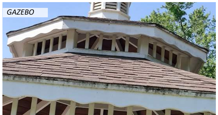
18 The painted wood base of the second roof tier is also showing signs of water damage
