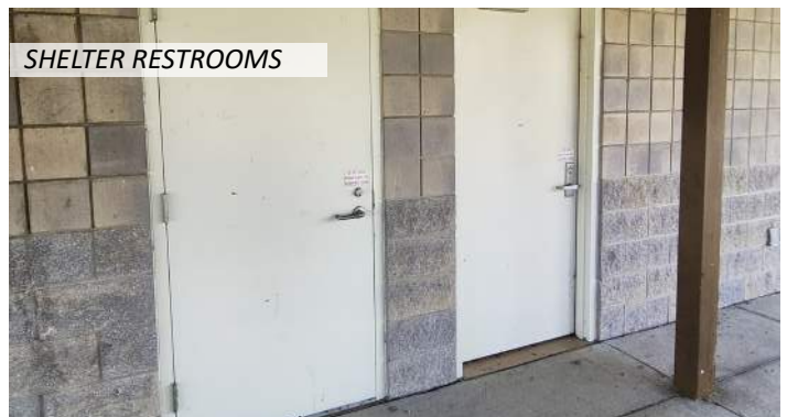
18 Entrance doors don't have correct accessible clearances
