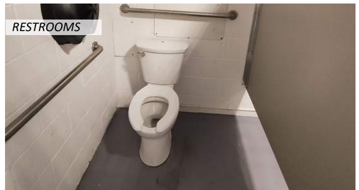
18 Accessible toilet stalls lack the correct clearance width and restrooms lack correct signage
