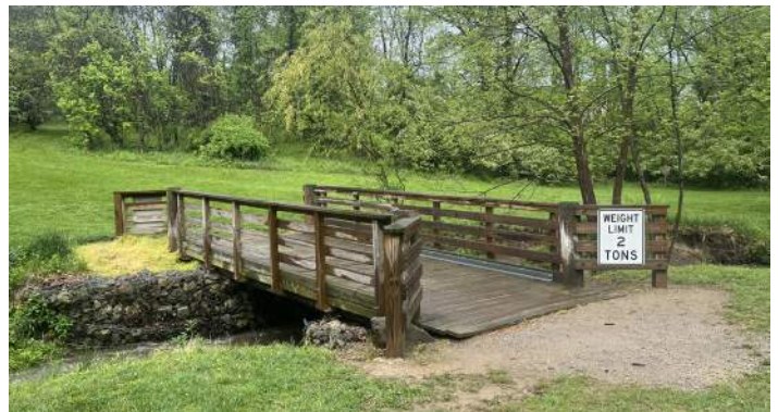
10 The bridge crossing the creek is slippery to cross and lacks a non-slip surface treatment
