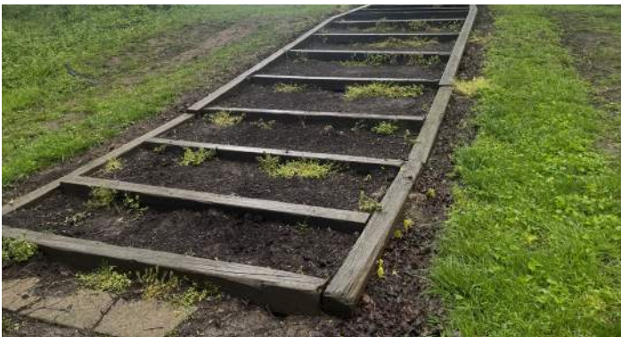
9 The stairs are heaving with eroded treads and are slippery when wet
