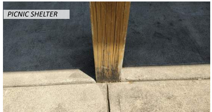
20 Minor stress cracks appear in columns, and there are signs of water damage at their bases
