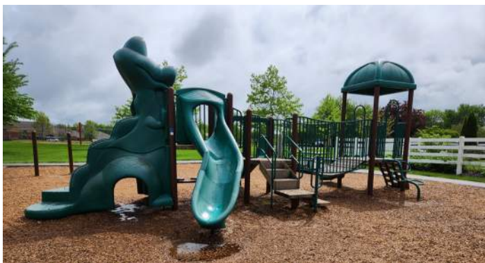
5 Playground appears aged and exhibits peeling, discoloration and some drainage issues
