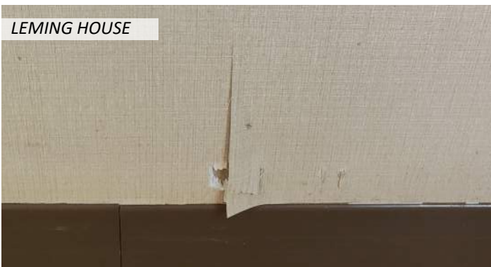
17 The gypsum soffits are cracking at the joints in several location and wallpaper is peeling
