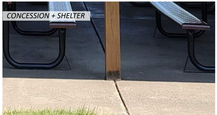
16 Wood columns show signs of minor water damage at the base and finish is weathering
