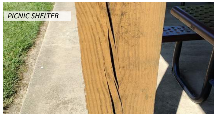
22 There are minor stress cracks in the wood columns and the wood finish is weathering
