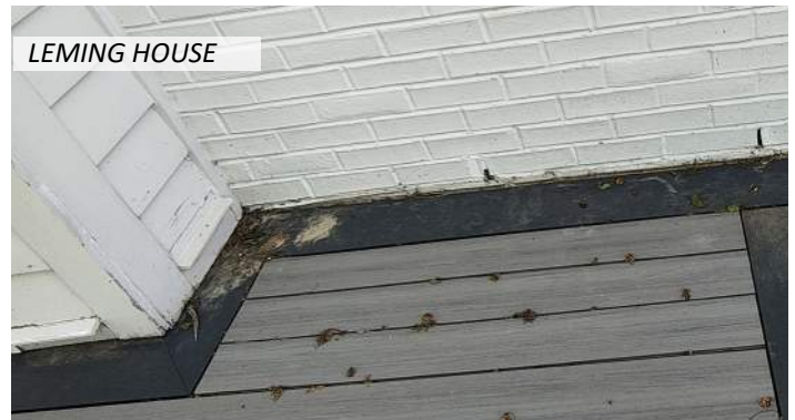
20 There is evidence of water damage at the building where it abuts the deck
