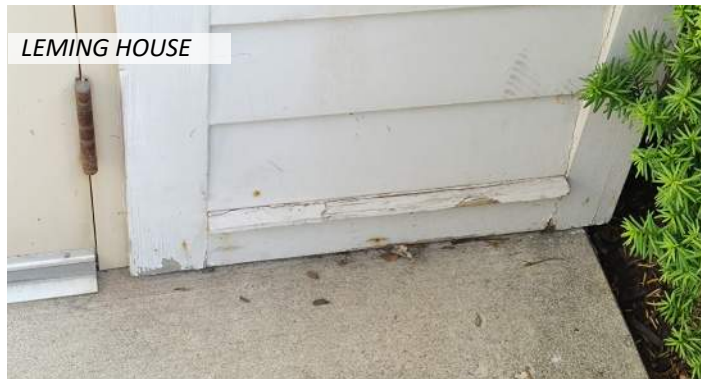
19 The wood drip edge at the windows and cladding base are all heavily deteriorated
