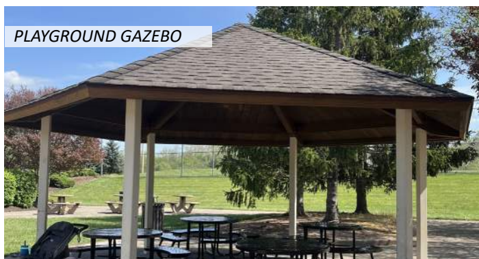
23 The metal columns and paint are in good condition but the wood finish is weathering
