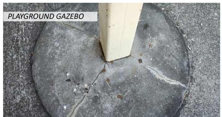
24 The concrete slab and footings are in fair condition, with minor cracks at the footings
