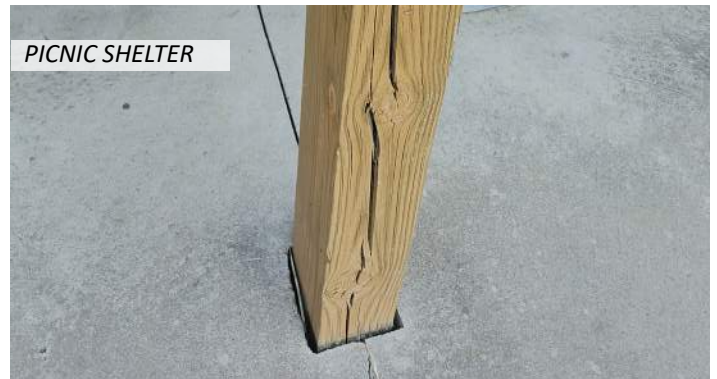
16 Minor stress cracks at some of the wood columns and the finish is beginning to weather
