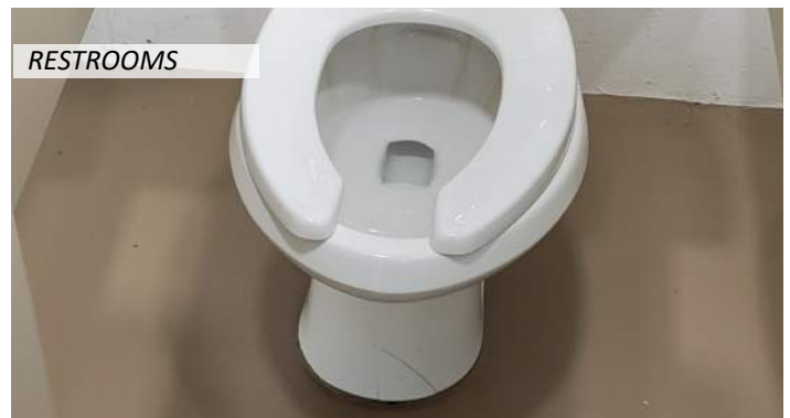
22 One toilet in women's restroom is cracked at the base and urinals lack accessible clearances
