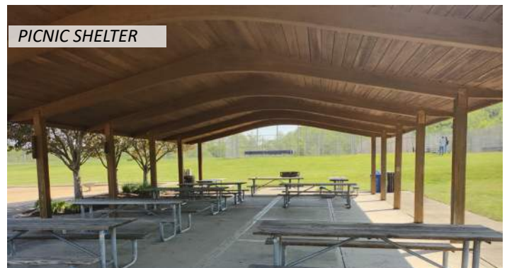
22 Some wood columns are starting to delaminate at the base and the wood is starting to weather
