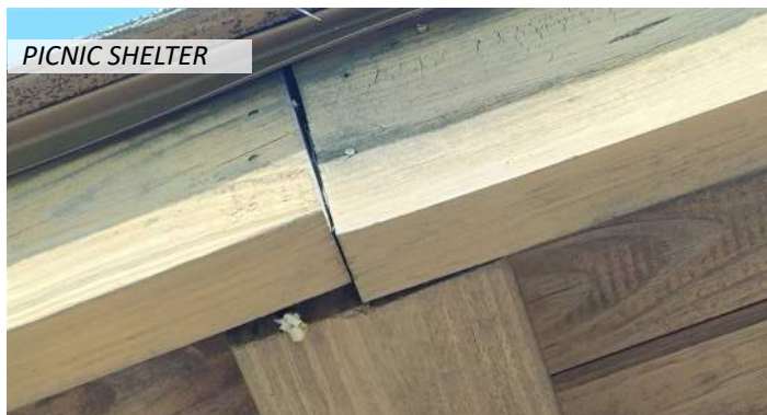
21 The painted metal drip edge is bent in some locations and the wood rakeboards are warped
