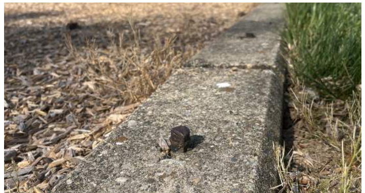
10 Rebar ties protruding from concrete border of playground
