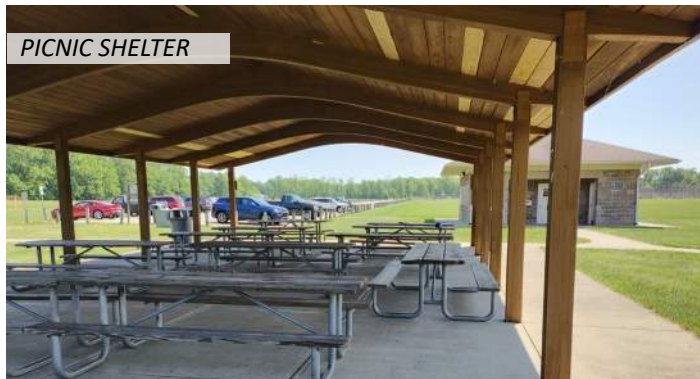
19 Roof, painted metal drip edge, and concrete pavers are in good condition
