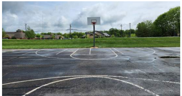
2 Basketball court is over striped on parking lot area, with surface cracking and seal coat wearing
